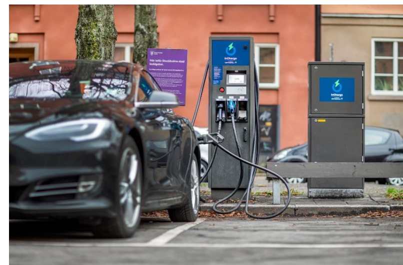
Fig.2 Charging Station in Sweden
